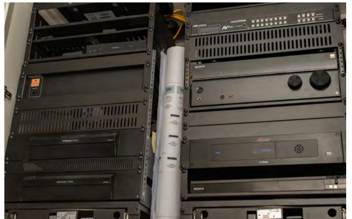
The James Loudspeaker M1000 DSP-enabled subwoofer amplifier resides with other electronics in the equipment rack
