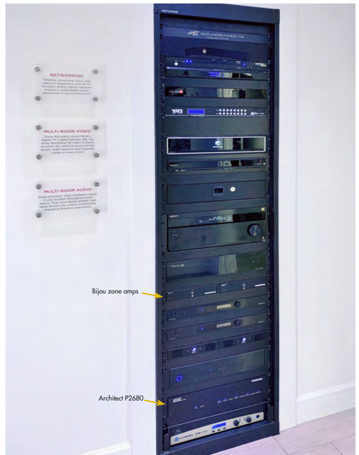
AudioControl Architect and Bijou amplifiers housed in a separate rack for the whole-house entertainment system
