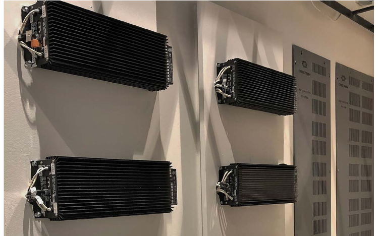
Crestron requested that the LumaStream power supplies be installed visibly so visitors to the showroom can fully understand the lighting technology
